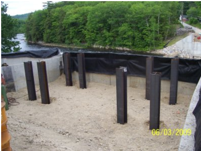
This is the construction of the temporary supports in the river for the placement of steel.
